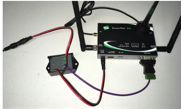
Watchdog installed on Cellular Gateway
